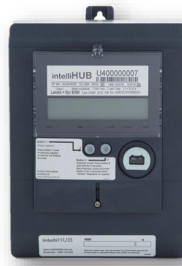
Three Element Meter and OP Controlled Load connected to C-Phase (i.e. General supply for 3 phase only or 2-Phase and OP)
